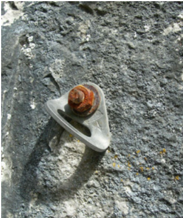
Galvanic corrosion between a stainless steel hanger and mild steel bolt causing the bolt to corrode.
