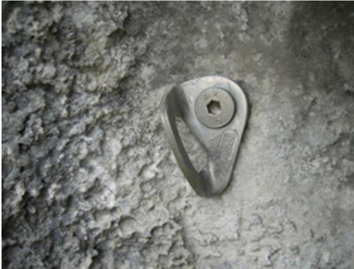
Sleeve anchor with a Petzl hanger.
